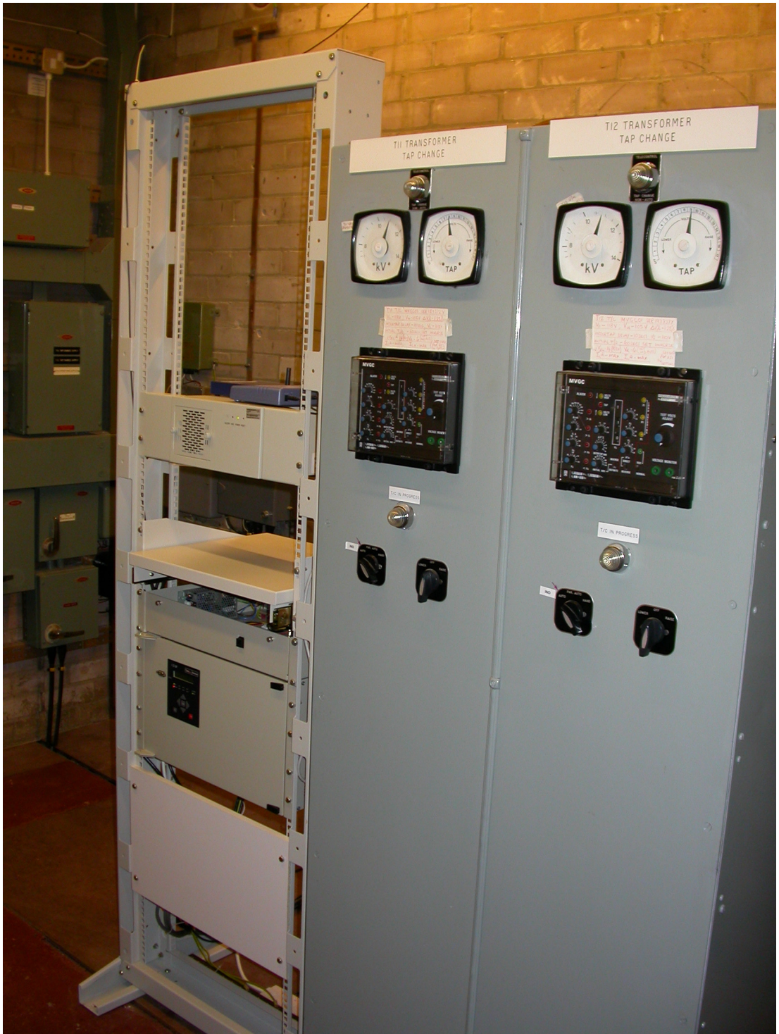
Figure 8 - GenAVC™ installation at Morton Park, adjacent to two Automatic Voltage Control (AVC) relays
