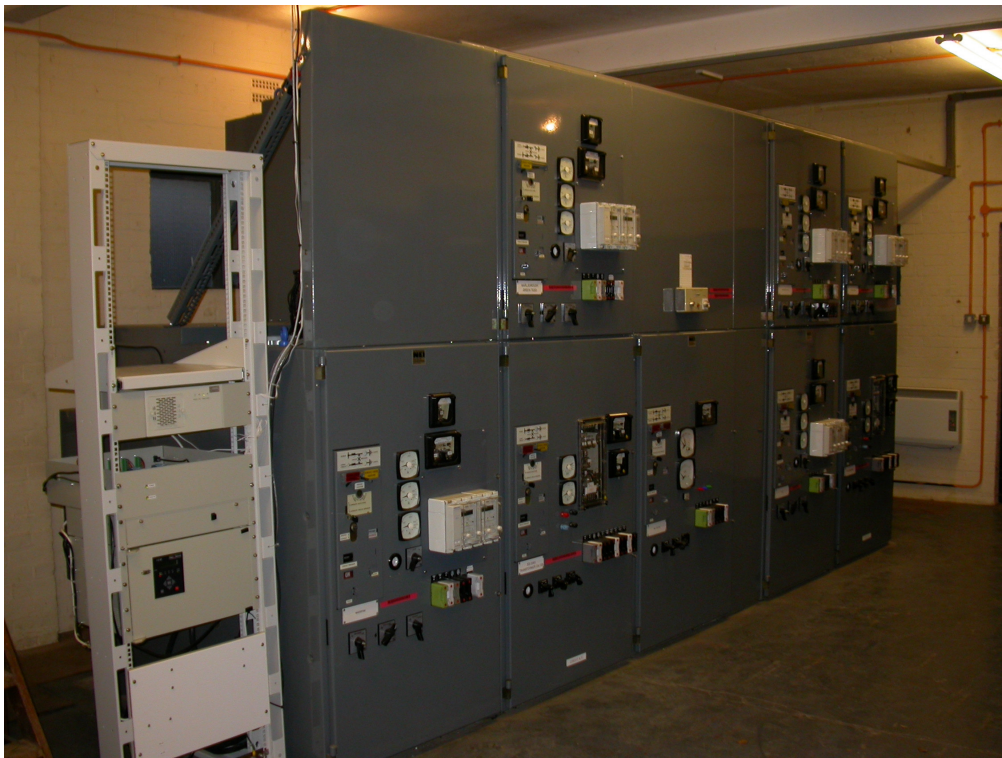
Figure 6 - GenAVC™ installation at Martham primary substation, adjacent to substation panels
