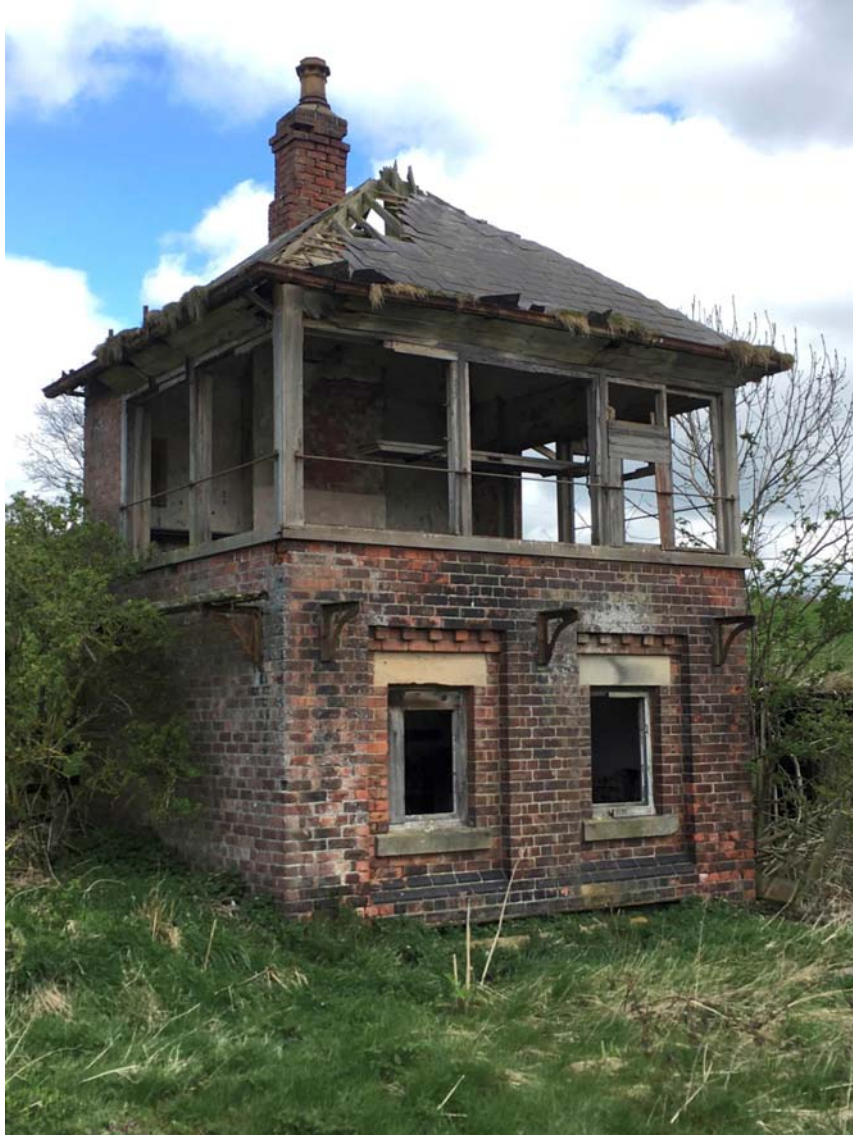
Figure 2: Broomielaw Signal Box (1897). Abandoned since 1965 and overall still structurally sound. Even the surviving timberwork, including block instrument shelf behind the front windows, is still potentially repairable and balcony ironmongery still extant.
