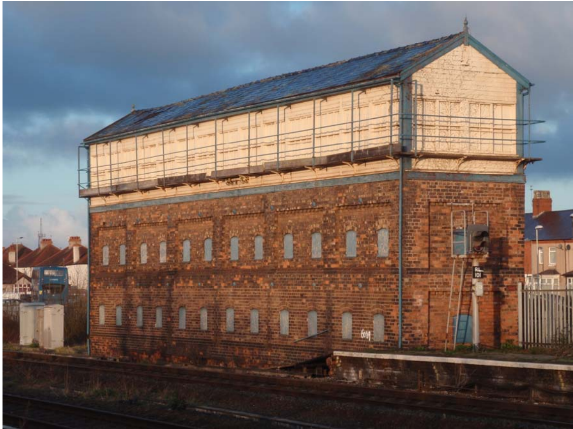
Figure 8: Rhyl No 2 Signal Box (1900). Although still structurally stable and reasonably carefully mothballed, the building presents a derelict impression.
