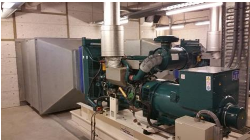
Figure 4: Diesel back-up generator in the JC Arena (photo by J.Warmerdam)
