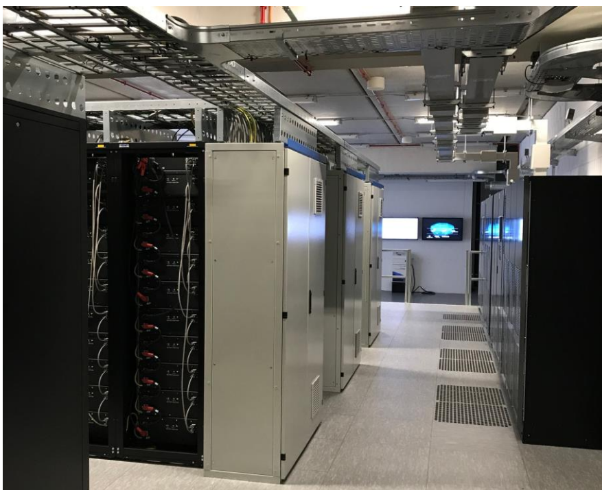
Figure 5: Part of the 3 MW battery system (photo by B. Jablonska).
