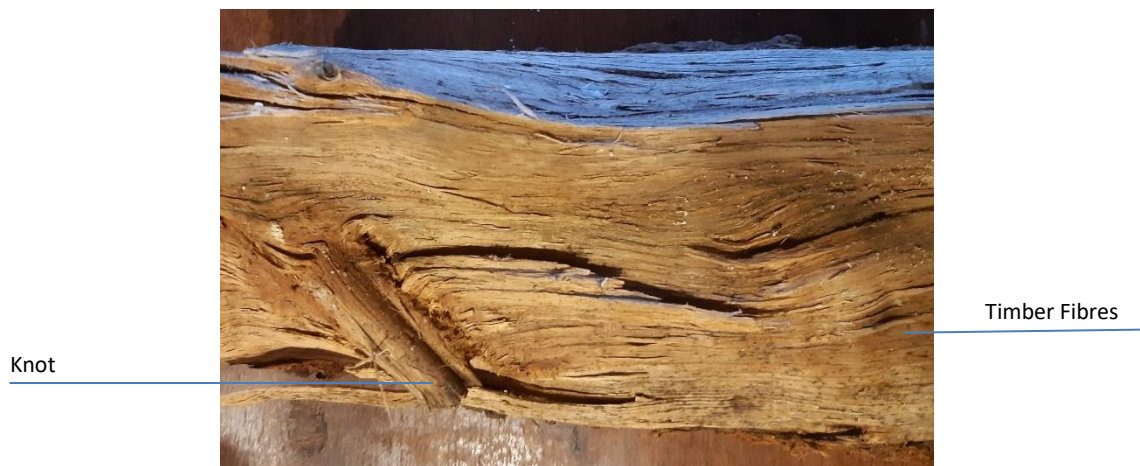
78 79 Figure 1. A section of a timber beam showing the devastating effect of a knot: it can be noted that timber 80 fibres are interrupted by the presence of a knot.
