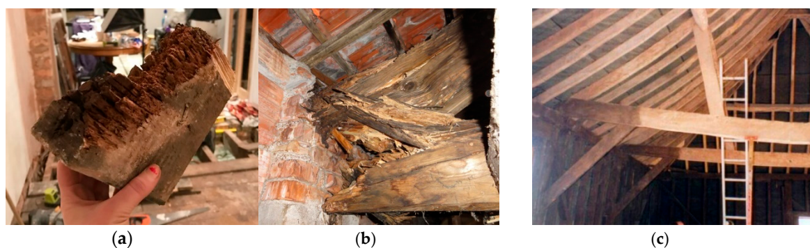
Figure 6. Examples of damage in timber structures: (a) and (b) Rotting wood at the beam-ends, and at the joists in timber roof truss; (c) Deformed timber tie in a frame of a roof structure because of over-loading.
