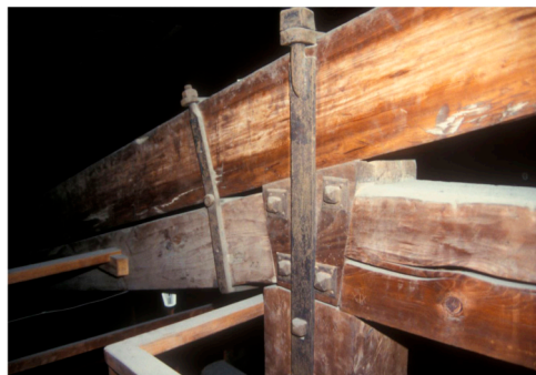
Figure 9. Salone dei Cinquecento, Palazzo Vecchio, Florence, Italy: Detail of timber roof structure and iron fasteners (the iron reinforcement is part of the original structure from 17th century).
