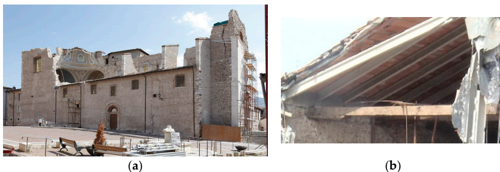
Figure 8. (a) St. Mary of Paganica ( S. Maria di Paganica in Italian) in L’Aquila after the 2009Abruzzo earthquake; (b) detail of the roof structure.
