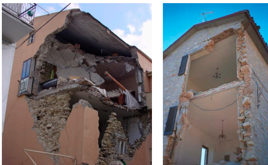
Figure 2. Examples of the effects of a typical intervention carried out in the 1980s in Italy: The intervention consisted of the removal of the timber-beam floor and roof, insertion of reinforced concrete (RC) ring beams, concrete-rib and hollow-block floor, RC slab roof.
