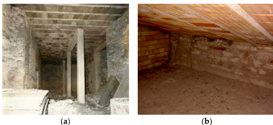
Figure 6. Example of an intervention carried out on a 14th-century building in Gubbio, Italy in the 1980s: (a) New RC frame, (b) replacement of timber-beam floor with a hollow-core concrete one.
