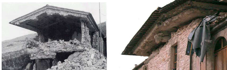
Figure 4. Examples of buildings where replacement of timber beam floor/roof was made (Umbria-Marche 1997 quake).
