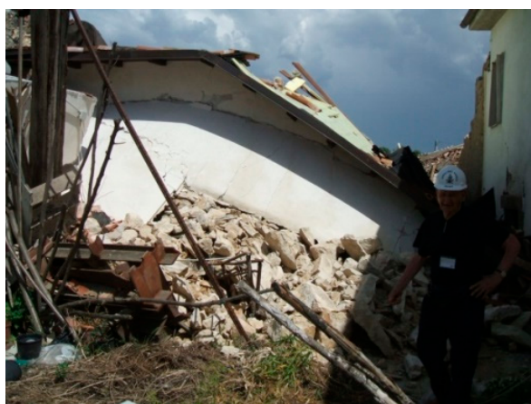
Figure 10. Example of ruined historic building with a portion of the façade wall left unreinforced (fair-faced aspect), without the application of RC jacketing.
