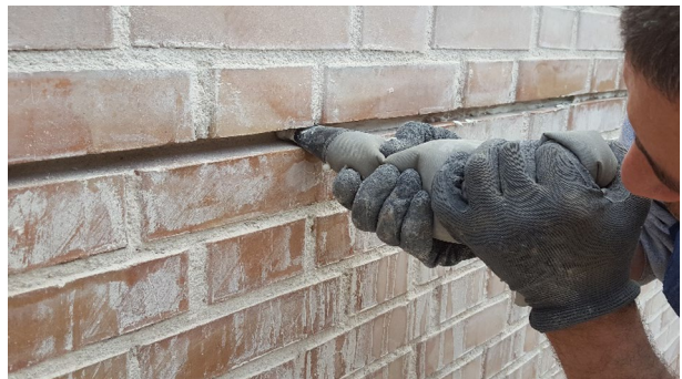
Fig. 9 A mastic gun was used before and after the application of the steel cable for joint repointing
