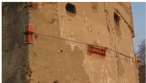
Fig. 1 An example of a provisional intervention aimed at preventing the out-of-plane rocking of the façade
