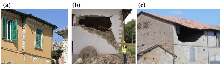
Fig. 14 Examples of out-of-plane mechanisms: a façade's out-of-plane rocking, b out-of-plane mechanism and shear/bending failure, c arch-mechanism
