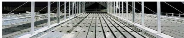
Figure 2.7 Linear Fresnel Reflector of the Power Plant [111]
