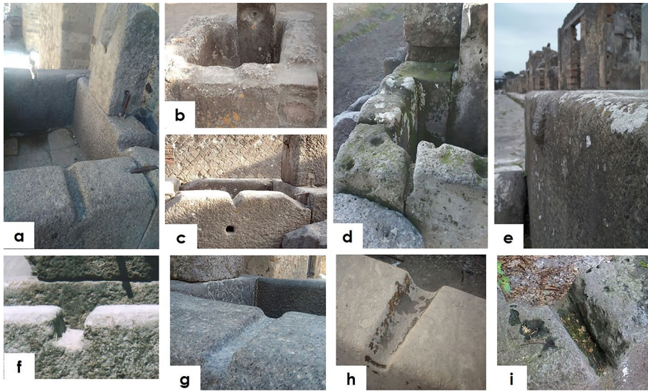
Fig. 5 Distinctive features of some overflow channels: a Fountain 24, with three overflow weirs; b Fountain 31, with a masonry basin presenting a large lowered front area; c Fountain 32 with an orifice lower than the original weir; d Fountain 37, with a gap between the two slabs at the front left in place of the regular channel; e Fountain 40, whose channel bottom is prolonged for 4 cm out from the side of the lacus ; f Fountain 13 overflow channel, with the largest rectangular cross-section; g Fountain 4 overflow channel, with a trapezoidal cross-section of minimum height; h Fountain 26 overflow channel, with neat edges (basin in travertine) and sides converging towards the outlet; i Fountain 37 overflow channel, with worn edges (basin in tufa)
