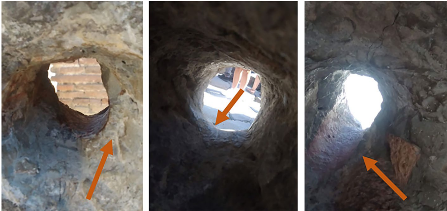
Fig. 8 Small portions of the lead supply pipes found attached to the sides of some spout orifices
