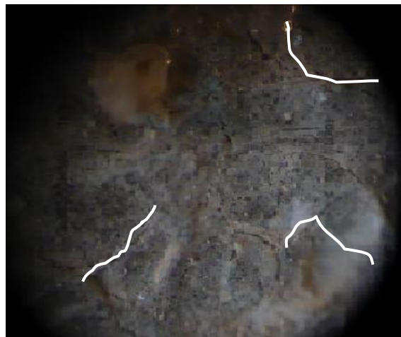
Figure 7 Shrinkage cracking on polypropylene fibre concrete
