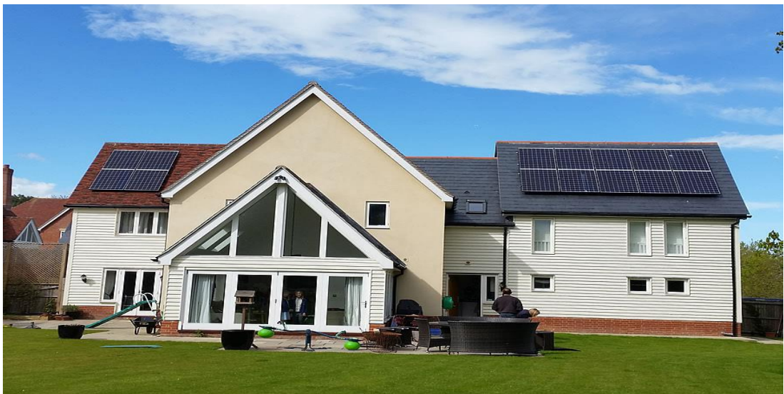
Figure 2.26 An installed photovoltaics rooftop in a retrofitted building (Chelsfieldsolar, 2018)
