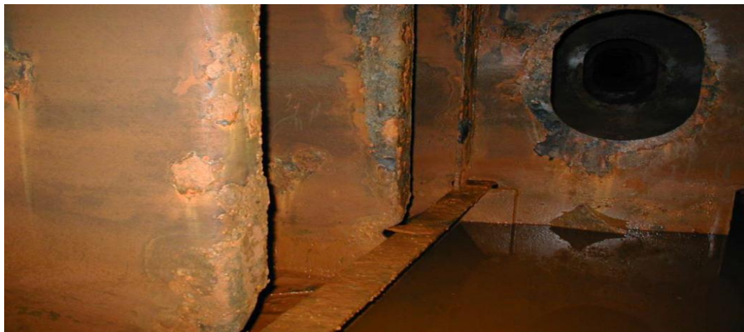
Figure 1 Accelerated corrosion following coating breakdown in WBT [8]
