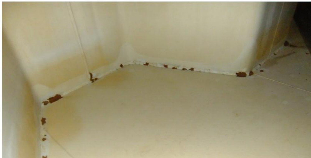
Figure 19 Pictorial view of coating failure at corners of WBT in-service
