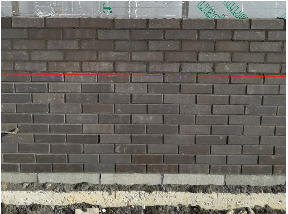
Figure 4.6 Brick wall before and after jointing (Photo taken by Orsolya Bokor in 2019)
