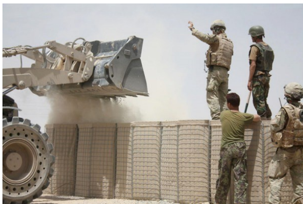
Fig. 1. Blast protection HESCO [9]
