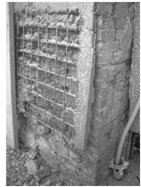
Figure 4 Failure of jacketing
