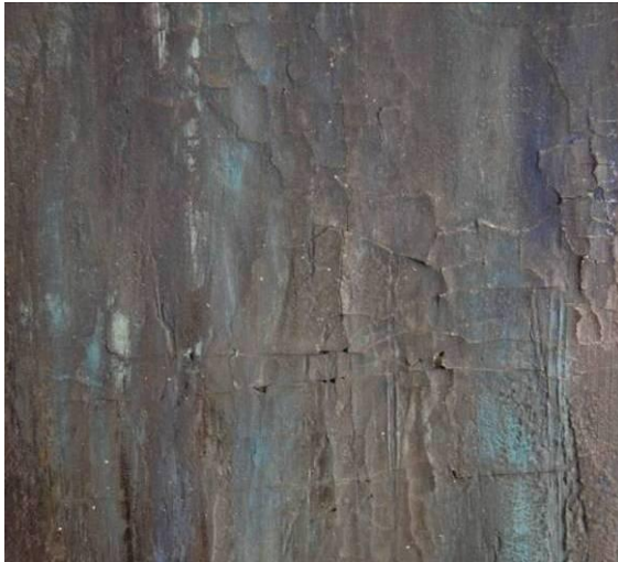
Figure E.06.1 Thick cracking paint in background
