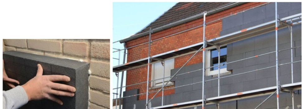
Fig. 2 Examples of “invasive” interventions aimed at reducing carbon emissions: the insulation coating covers the historic brickwork masonry and its architectural decorations
